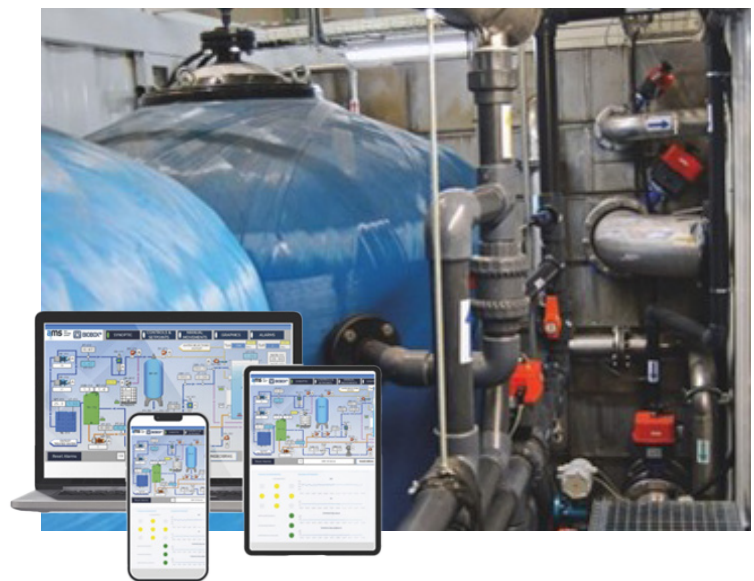
Figure 3: BIOBOX® Nitrate Systems Include 100% Automation and 24/7 remote monitoring and control
