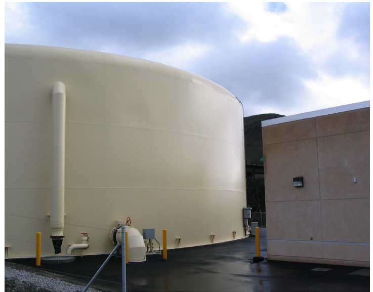
2 MGD storage facility (Clearwell #2) at San Luis Obispo Water Treatment Plant where the online THM-100 is used to control the THM removal equipment.
