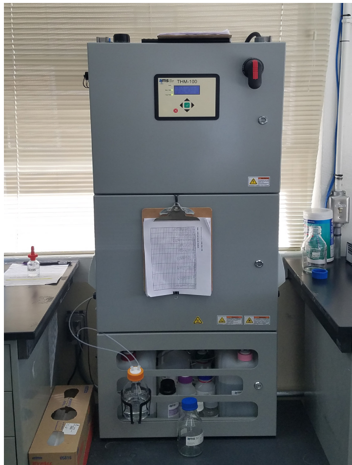
Online THM-100 analyzer installed at the onsite laboratory of the San Luis Obispo Water Treatment Plant.
