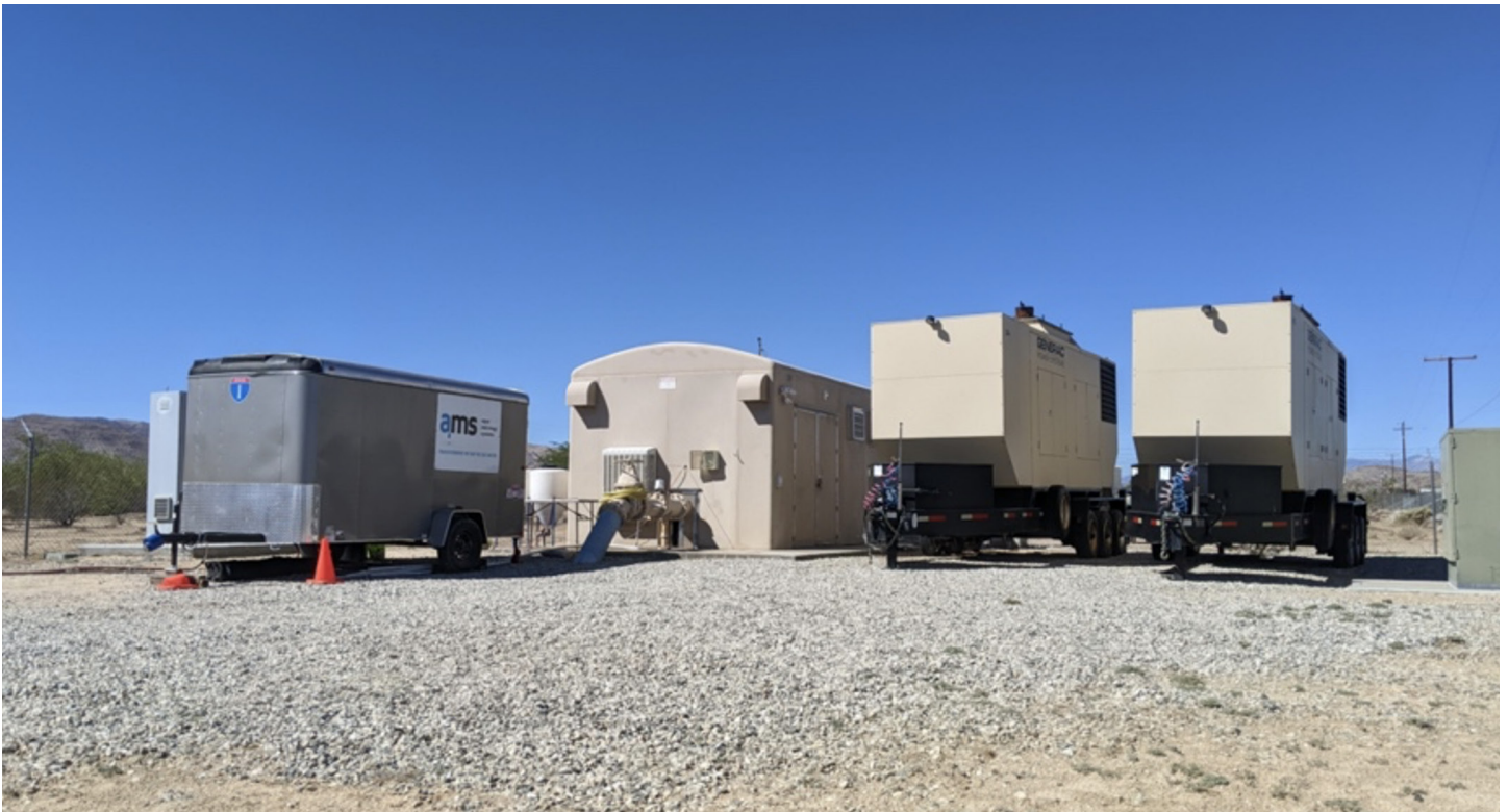
Figure 1. SafeGuard™ H2O Cr6 Removal Demonstration Trailer at Joshua Basin Water District. The demonstration system was comprised of five main components: the stannous reagent generation control module, electrolytic reagent generator, contactor, sand media filter and the MetalGuard™ online Cr6 monitor.
