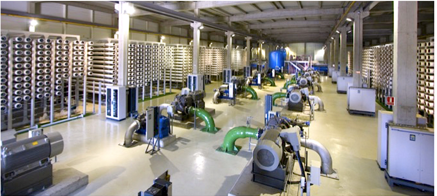
Figure 1. RO Membrane System at Sant Joan Despí DWTP
