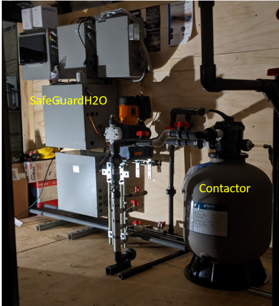
Figure 2 - SafeGuard™ H2O Trailer Mounted Arsenic Removal Demonstration System Installed at Isleton Well #3A
