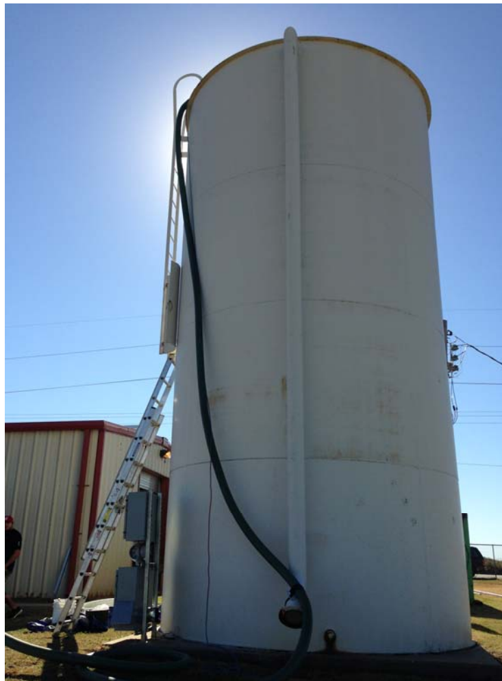
Figure 2-3 OMT WTP Clearwell
