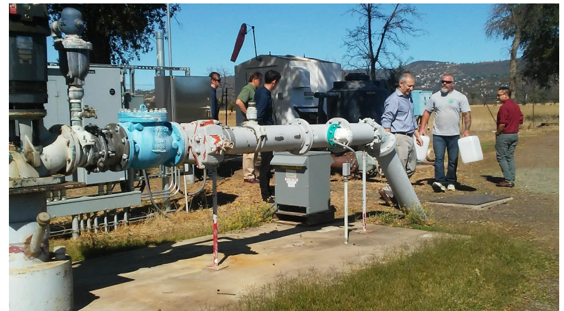
SafeGuard™ H 2 O Cr(VI) remediation system pilot demonstration at Hidden Valley Lake Community Services District
