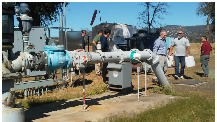
AMS pilot demonstration of its SafeGuard™ H2O Hexavalent Chromium [Cr (VI)] remediation system at California's Hidden Valley Lake Community Services District.
