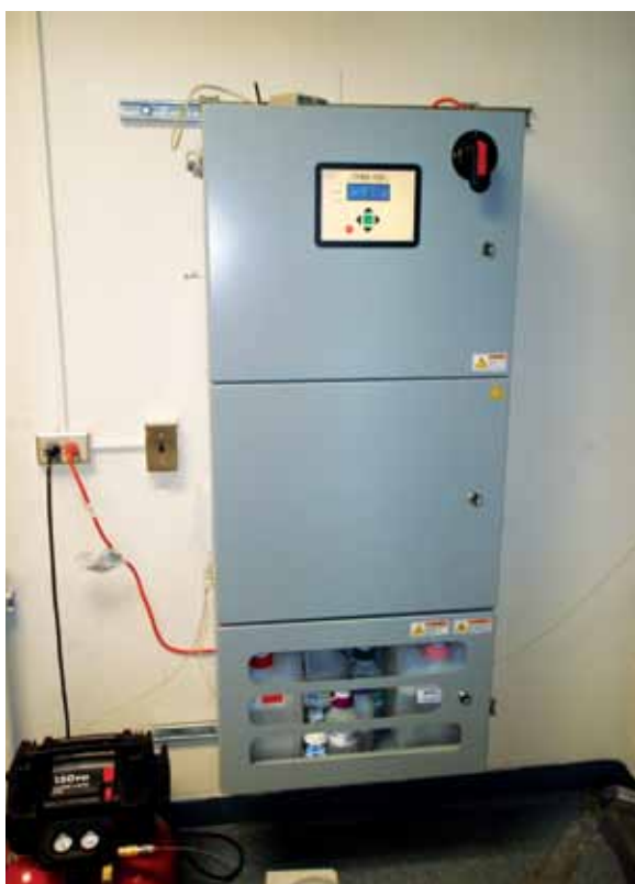
A THM analyzer was installed to monitor the THM levels of the incoming water from the Middlesex Water Co. as well as the THM levels of the water leaving the tank.
